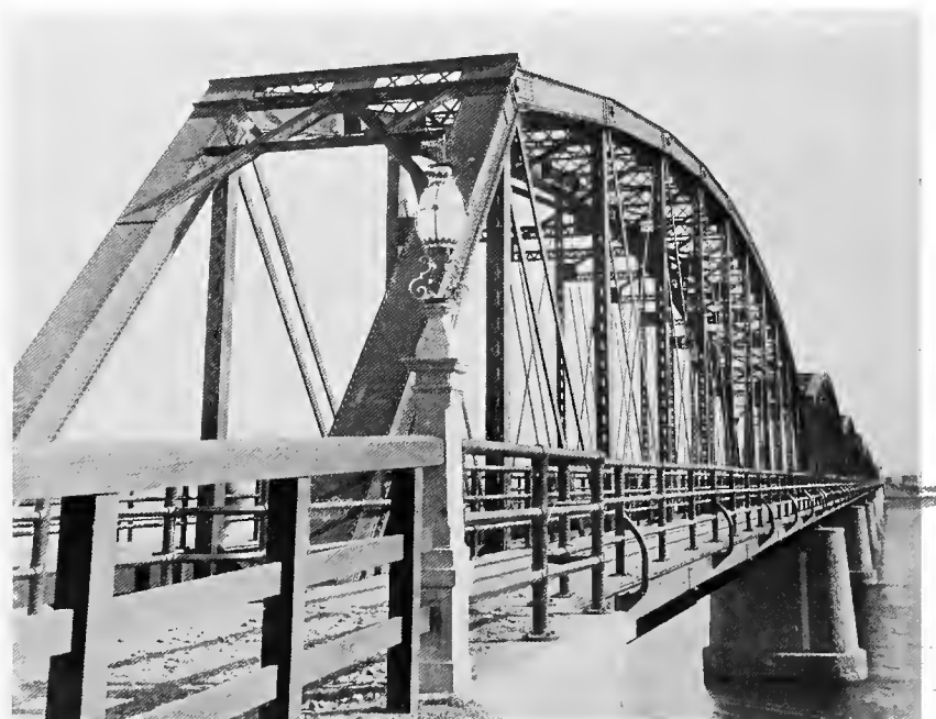
The great steel bridge across the Yalu River at Antung, connecting the South Manchuria Railway and the Chosen State Railways
